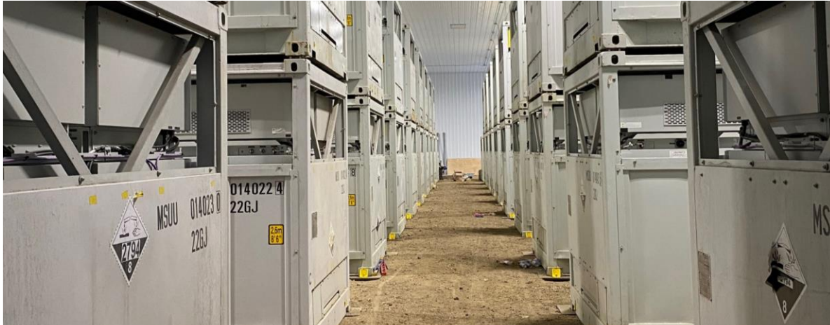
CANADA'S LARGEST VANADIUM FLOW BATTERY Solar plus Storage 8.4MWh
