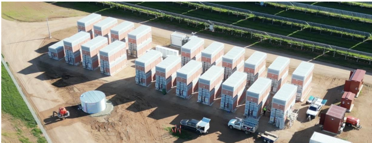
AUSTRALIA'S FIRST DISPATCHABLE SOLAR PLANT Solar plus Storage 8.3 MWh
