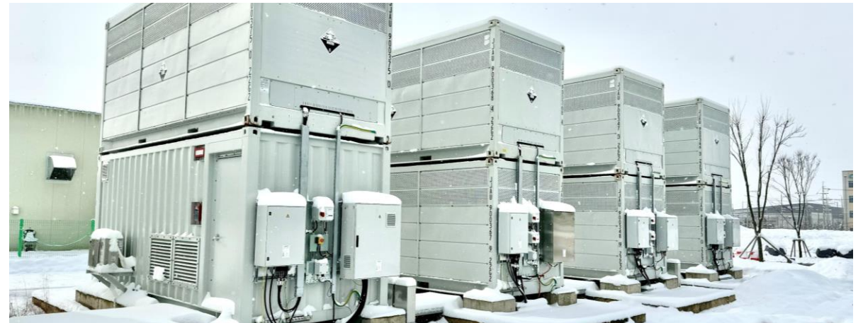
HIGH THROUGHPUT DEMONSTRATOR / KEPCO Grid Services 1.5 MWh
