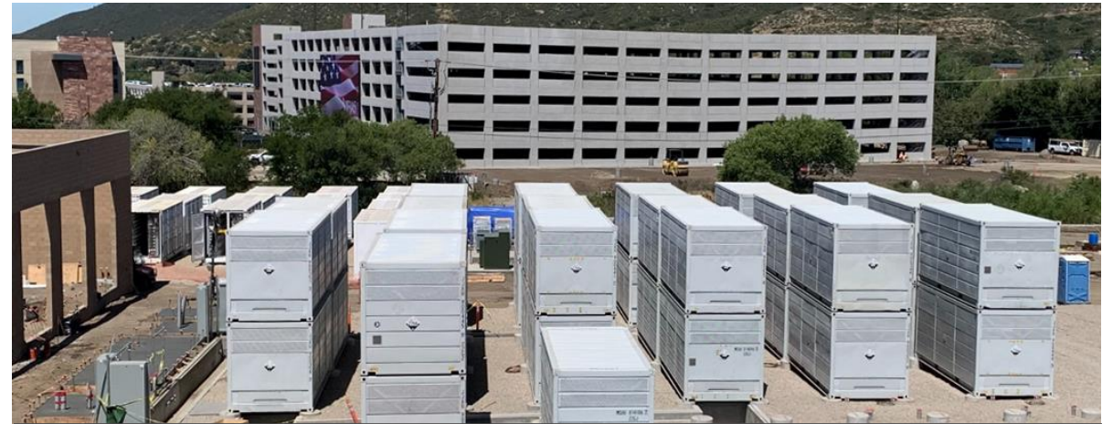
NORTH AMERICA'S LARGEST VANADIUM FLOW BATTERY / California Microgrid Resilience 10 MWh
