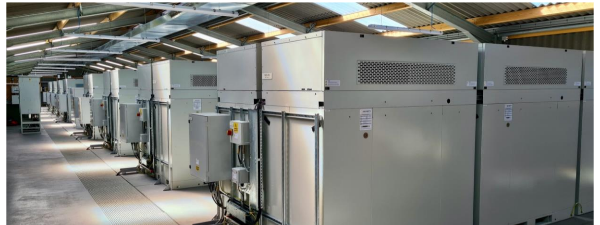
EUROPEAN MARINE ENERGY CENTER / Scotland Dispatch 1.8 MWh
